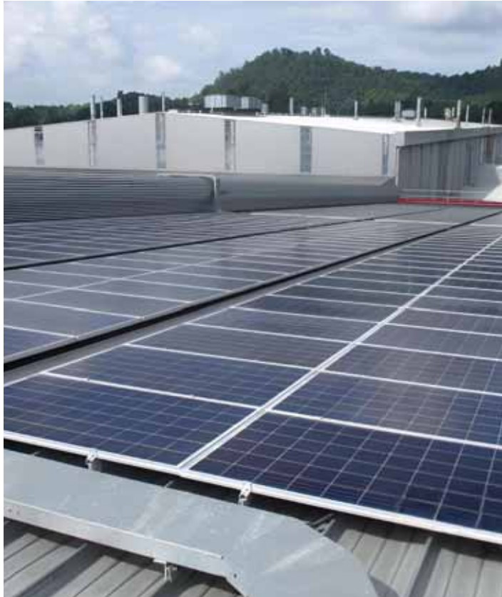
Rooftop solar panel system is the Group's continuous efforts in reducing carbon footprints.
