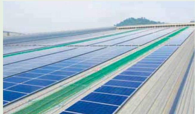
An aerial view of solar panel roof
