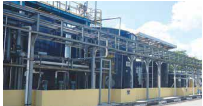
Waste water treatment plant
